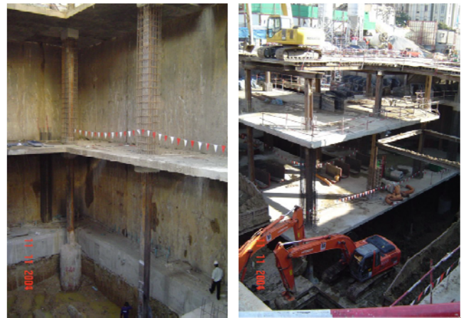
Figure 9 Application of top-down method for deep excavation work in Bangkok (Thasnanipan et al., 2006)
