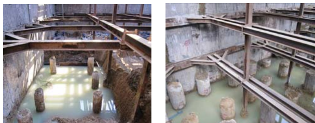
Figure 16 Groundwater encountered in basement excavations deeper than -17.50m
